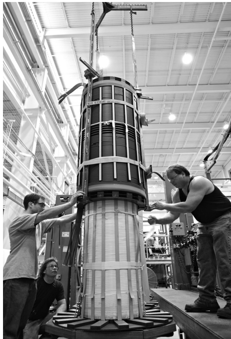
FIGURE 2.8 Concentric arrangement, outer coil being lowered onto core leg over top of inner coil.
