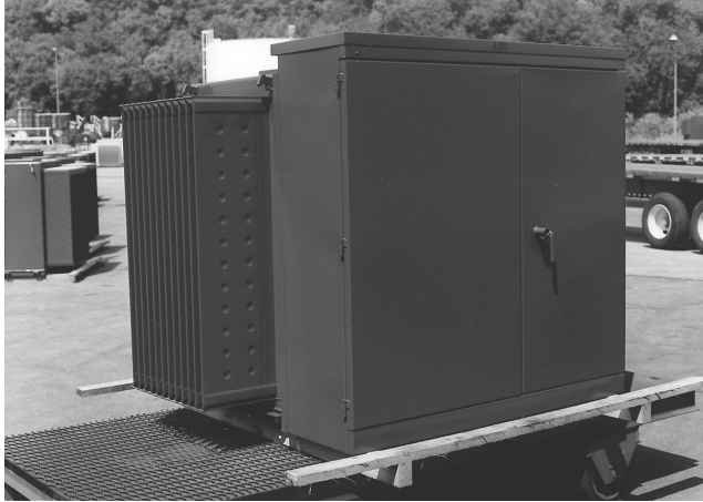
FIGURE 3.2 Typical three-phase pad-mounted distribution transformer. (By permission of ABB Inc., Jefferson City, MO.)
